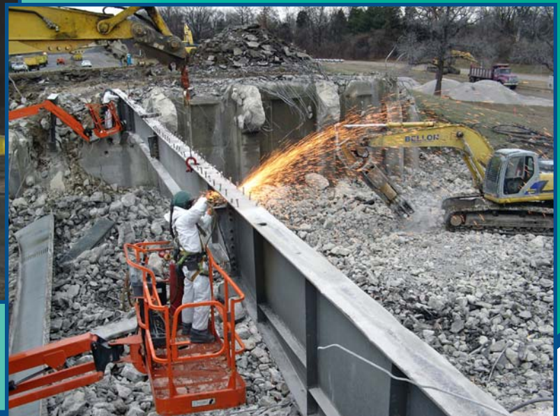
BELOW: An iron worker uses a cutting torch to remove a steel beam from the rubble of the bridge.
