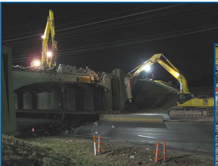
ABOVE: The I-64 bridge over Lindbergh Boulevard was the first to be demolished just two days after the highway was closed.
